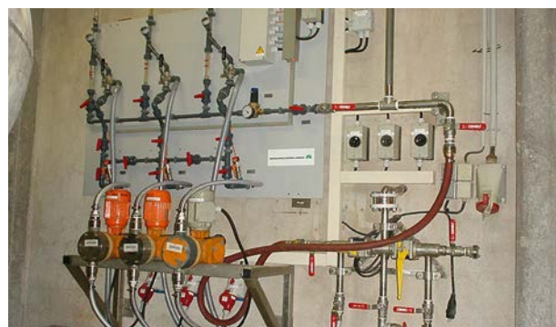
Figure | Defoamer dosage system
