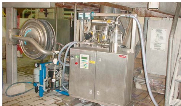
Figure | Gas Analyzing System Mütek Gas 60
